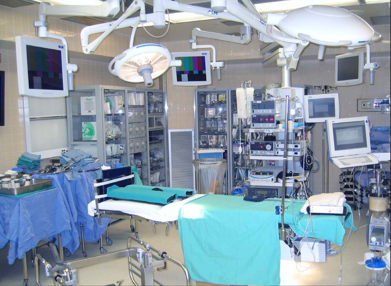
The OR of the Future at Massachusetts General Hospital in Boston includes a wide array of medical devices.
